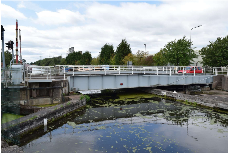
Plate 13: View north-east across the swing bridge at the west end of Keadby Lock [NHLE1005204; NHLE1342734], with Keadby 1 Power Station in the background.
