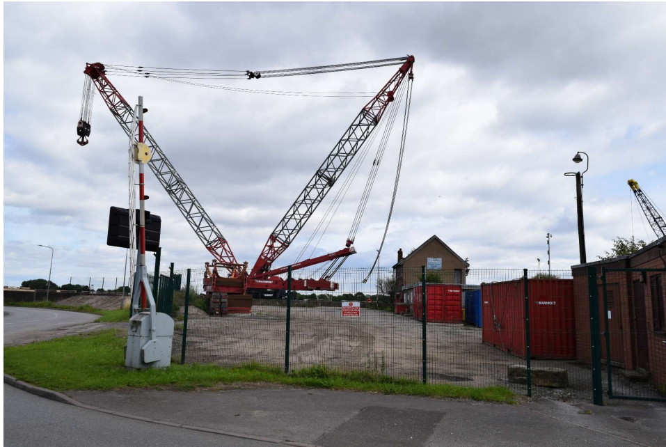
Plate 11: Area of concrete hardstanding with large crane preset (Waterborne Transport Offloading Area), to the north side of Keadby Lock [NHLE1005204; NHLE1342734], looking east.
