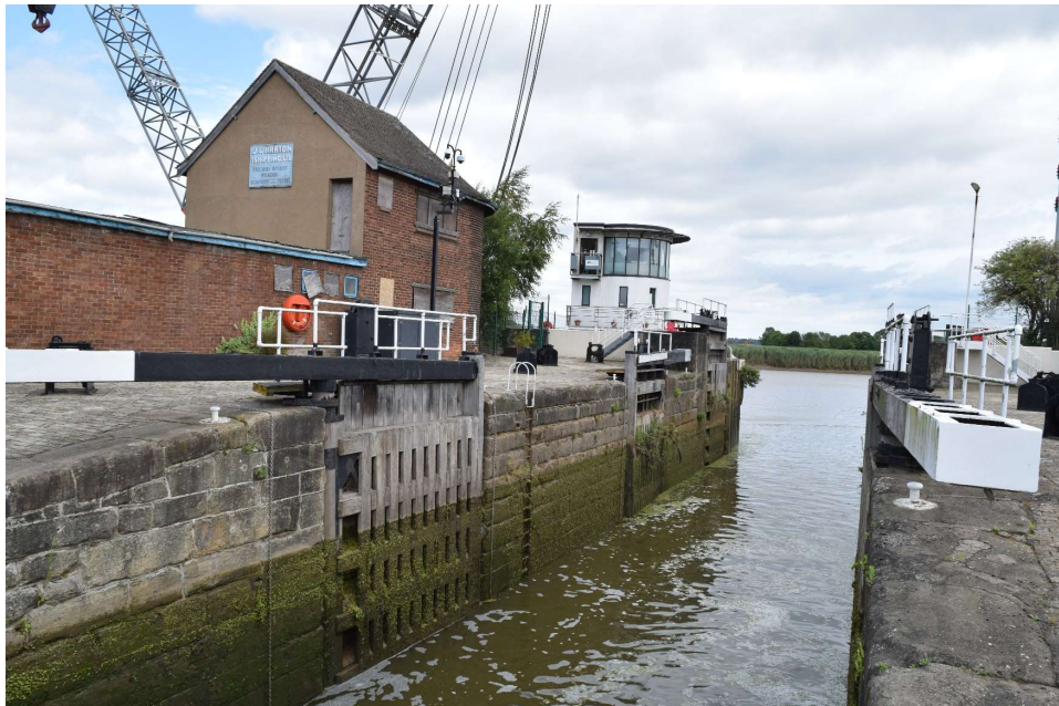
Plate 10: View east along Keadby Lock [NHLE1005204; NHLE1342734] at its exit to the River Trent.
